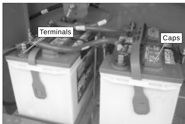
Figure 7.6 – Emergency Power Battery
