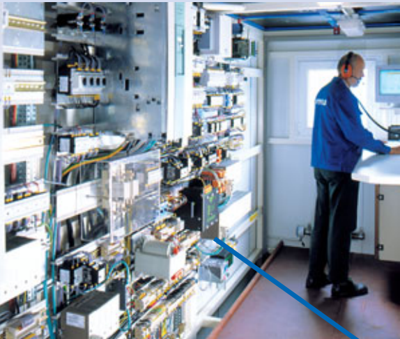
Air-conditioned electrics compartment
