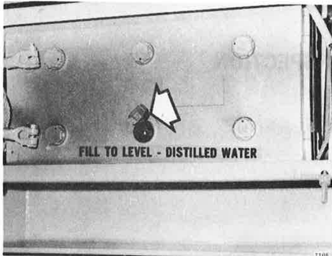
Figure 82 ELECTRICAL STORAGE BATTERY
