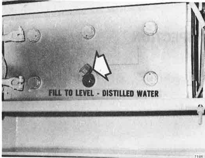
Figure 82 ELECTRICAL STORAGE BATTERY
